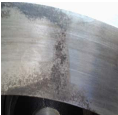
-Crevice & Galvanic corrosion
